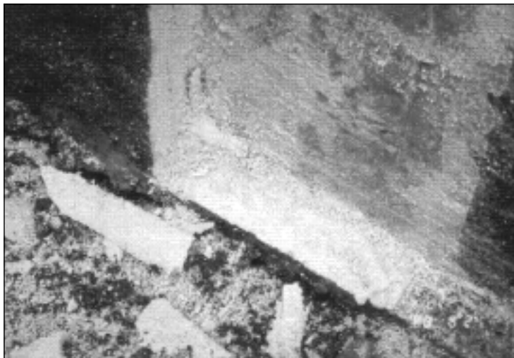
Figure 8. The spray-polyurethane foam bonded well to the concrete wall and footing. Remnants of the product still bonded to the concrete can be seen here.
