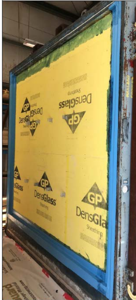
Photo I1 – Opaque steel stud with foundation interface wall section; wall perimeter prepared with membrane and brick ties sealed with sealant prior to product application
