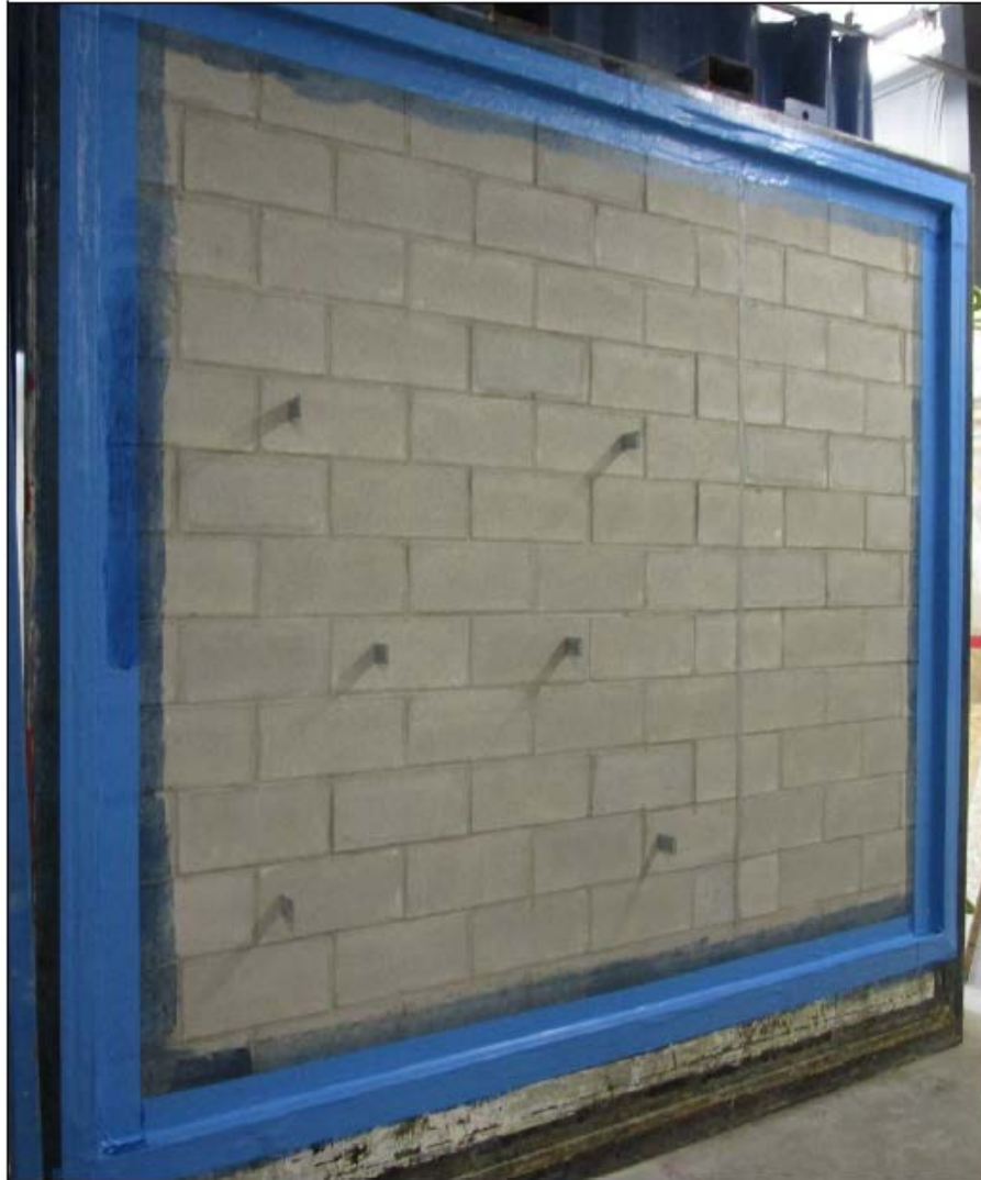
Photo L1 – Penetrations wall section; wall perimeter and foundation interface prepared with membrane and prior to product application
