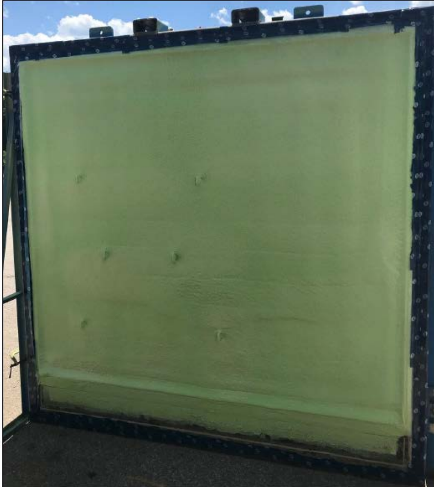
Photo I2 – Air barrier applied onto CMU wall (typical wall and not actual representation)
