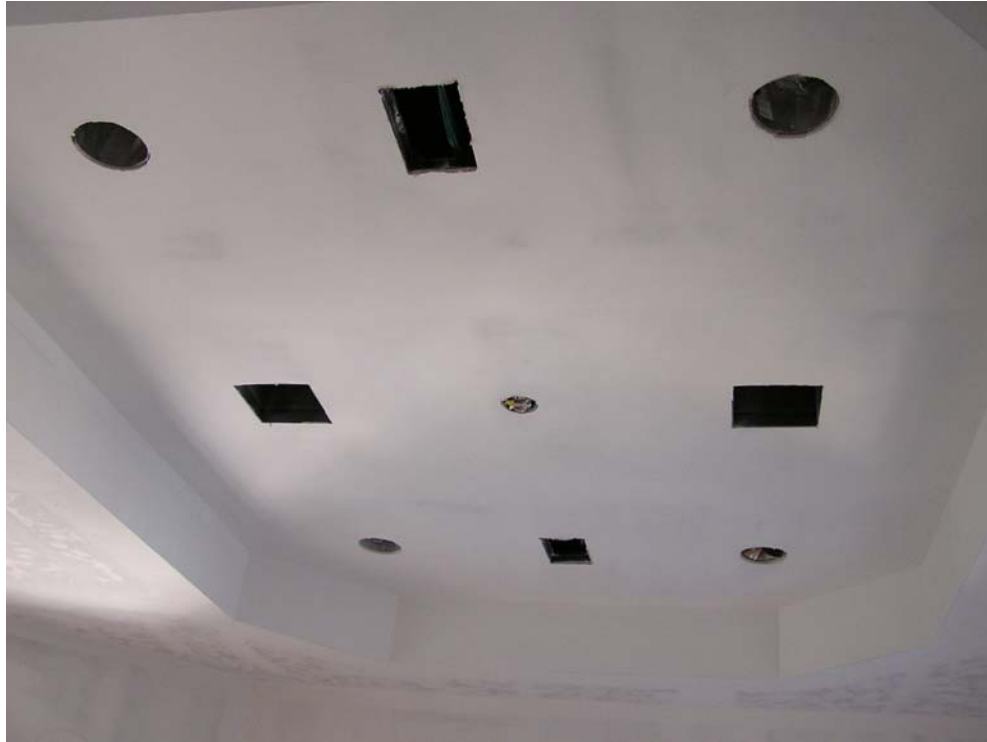
Photograph 1: Ceiling Penetrations – “Swiss Cheese Services”
